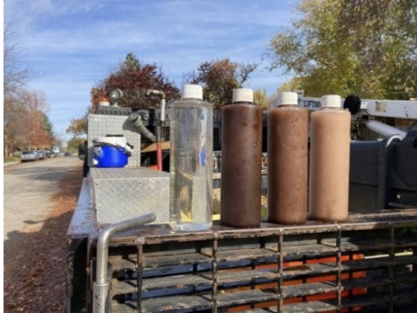
Image courtesy of American Pipeline Solutions (Left) After, (Middle) During, (Right) Before Ice Pigging
