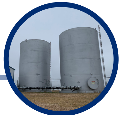
Step 3: Storage Tank
