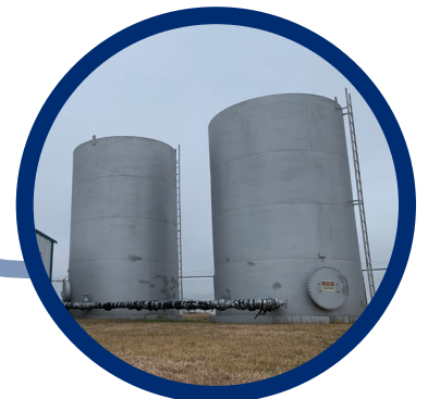
Step 3: Storage Tank
