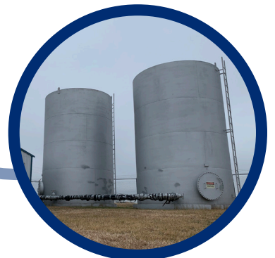
Step 3: Storage Tank
